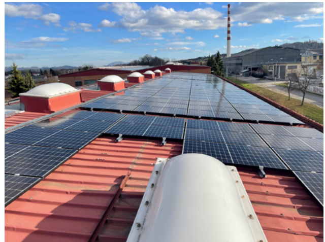
The solar power plant installed on the Polimeri facilities. Installed power 492.75 kWp, planned production 542 MWh
