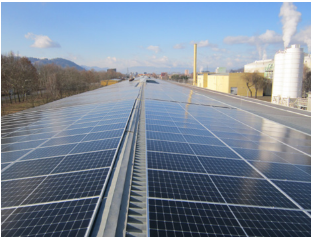
A solar power plant installed on the Valjarna building. Installed power 999.8 kWp, expected production 1,099.78 MWh.
